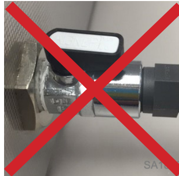
Drain Valve Open
